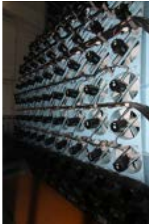
(A) Wall of fans.
