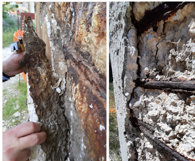
FIGURE 2 Examples of deterioration penetration beyond external surface, sometimes observed under severe corrosion.
