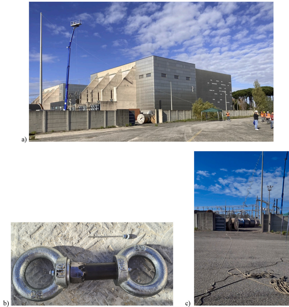
Fig. 1. Live cable (a), specimen for the release and the metal bar broken after the test (b); released cable (c).
