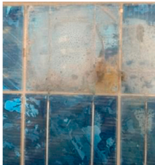
Figure 14. Advanced glass corrosion across a PV module surface, showing widespread hazing and opacity caused by environmental exposure. The affected area exhibits reduced transparency and transmission loss, likely due to degradation of anti-reflective coatings and chemical interactions with atmospheric pollutants [74].
