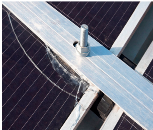
Figure 10. Example of glass breakage on a PV module caused by mechanical mounting stress (adapted from [70]).
