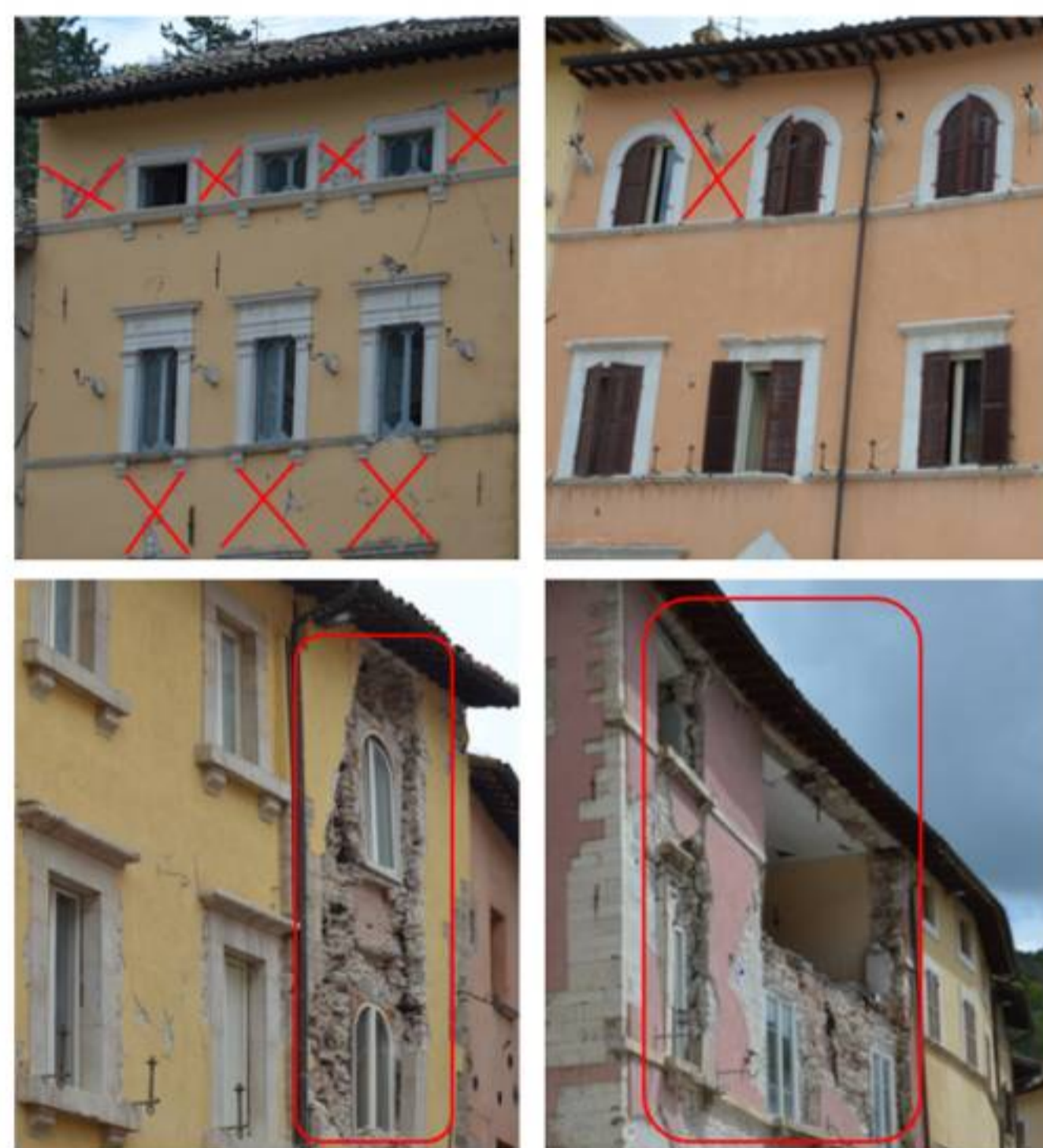
Fig. 6. Examples of damage in the historic center of Visso. Cracks IP are marked with X, while OOP activations are circled.
