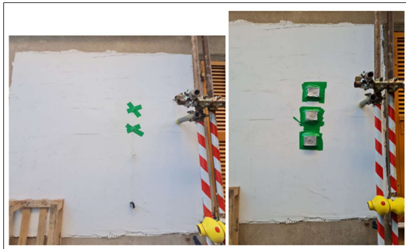
Figure 7. HFM installation to measure the contribution of the nanotechnological mortar. Outside view, two years after the end of the installation cycle.
