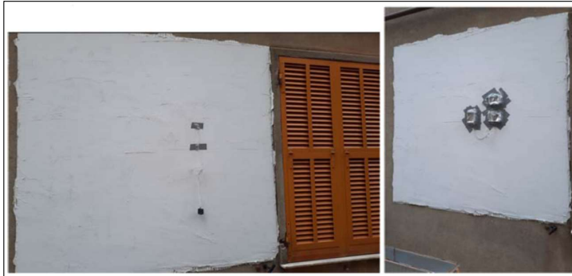
Figure 6. HFM installation to measure the contribution of the nanotechnological mortar. Outside view, just after the end of the installation cycle.
