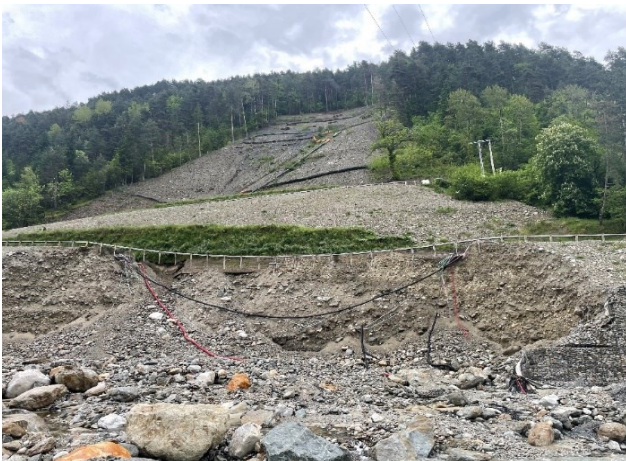
Figure 26: Municipality Road collapse due to a flow slide occurred during Alex storm
