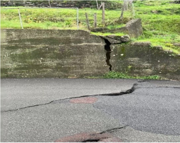
Figure 89: Retaining wall split (1)
