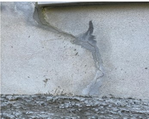
Figure 84: The damage on the exposed asset's wall (2)
