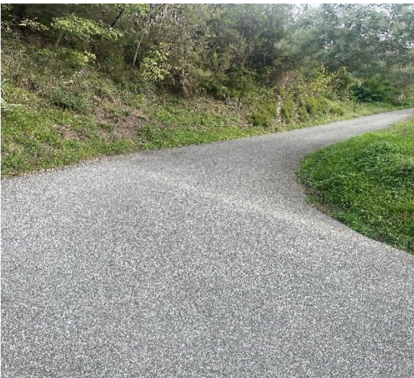
Figure 85: A road detail inside the dormant landslide (3)
