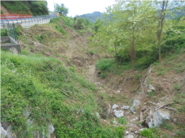
Figure 16: The Rio Vignale River erosion and the retaining wall (2019)
