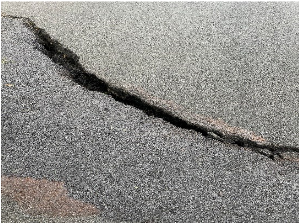
Figure 90: The road failure (2)
