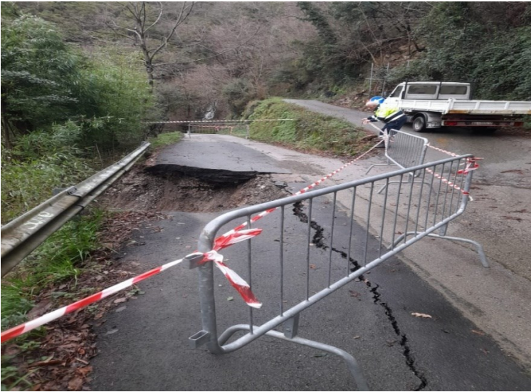
Figure 9: Municipal Road destruction by a terrain sliding effect in San Colombano Certenoli Municipality
