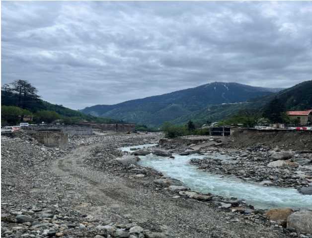
Figure 27: Roadway bridge detriment due to the water speed and intensity of Vésubie river
