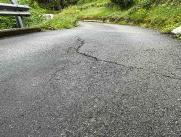
Figure 83: The surficial fracture on the road (1)
