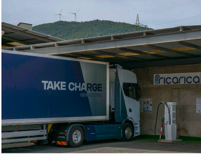
Fig. 1. The Fera Windfarm and the Ricarica EV chargers.
