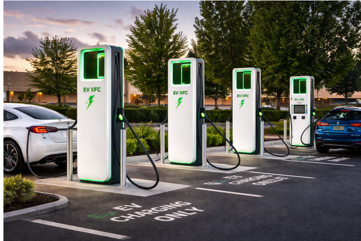
Figure 1.2: Extreme Fast Charging Station
