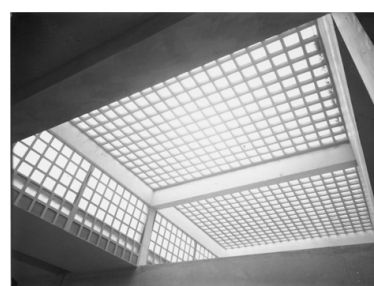
Fig. 6 – In this vintage photo it is possible to notice the difference between the colour of the skylight structural elements and of the underlying beams (Terragni's Archive, 1936)
