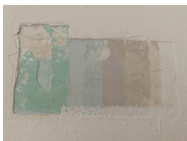
Fig. 4 – Stratigraphy of finishing layers on the ground floor (Photo by Sara Mauri, 2016)
