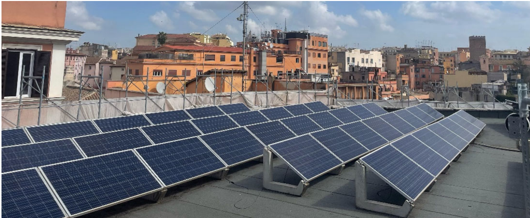
Figure 7. Lab’s rooftop photovoltaic system.
