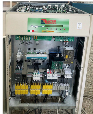
Figure 10. Three-phase bidirectional inverter connected to Flex'Ion battery.
