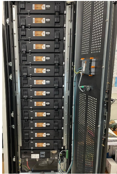
Figure 9. SAFT Flex'Ion 23 MFe storage system.
