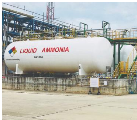
Figure 47: Type C tank for storing liquid ammonia
