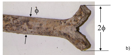
Fig. 12. Fish-tailed anchorage of bending reinforcement. From a residential building in Genoa, Villa Grüber park, Genoa, Porcheddu Building Company, in-between 1920-to-1930. Main geometric dimensions.
