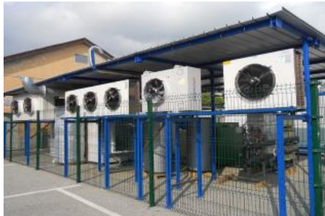
Figure 52 Savona Campus Laboratories thermal dissipators
