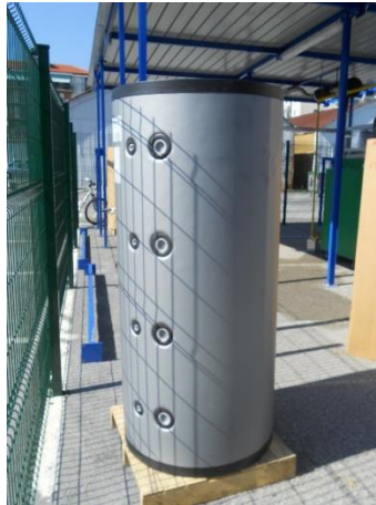
Figure 49 500 litres Thermal Energy Storage in Savona Campus
