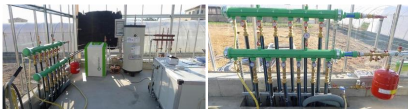
Figure 4.6 – Geothermal heat pump and geothermal probes in the greenhouse
