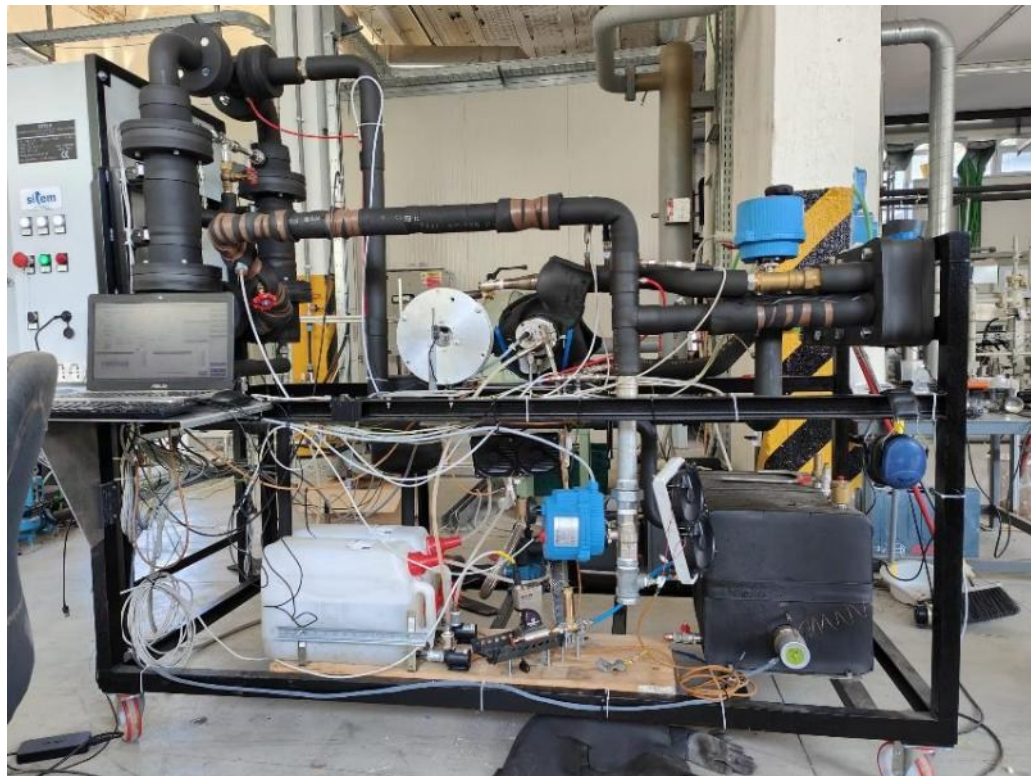
Figure 70 – Overview of the emulator plant in its final configuration.
